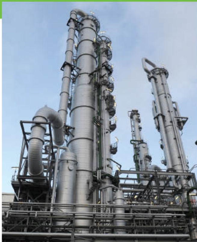
HPPO plant in Antwerp, Belgium
